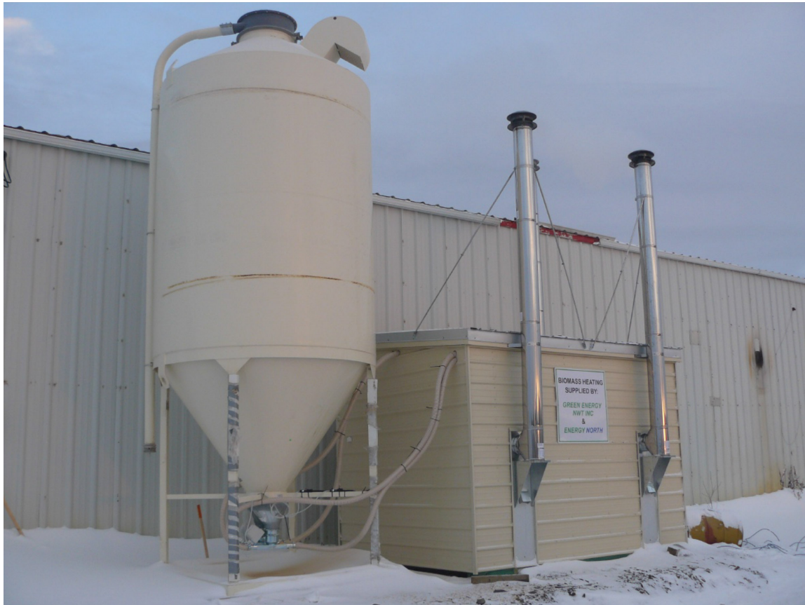
Figure 7: Exterior boiler room housing a two-boiler cascade in Norman Wells
