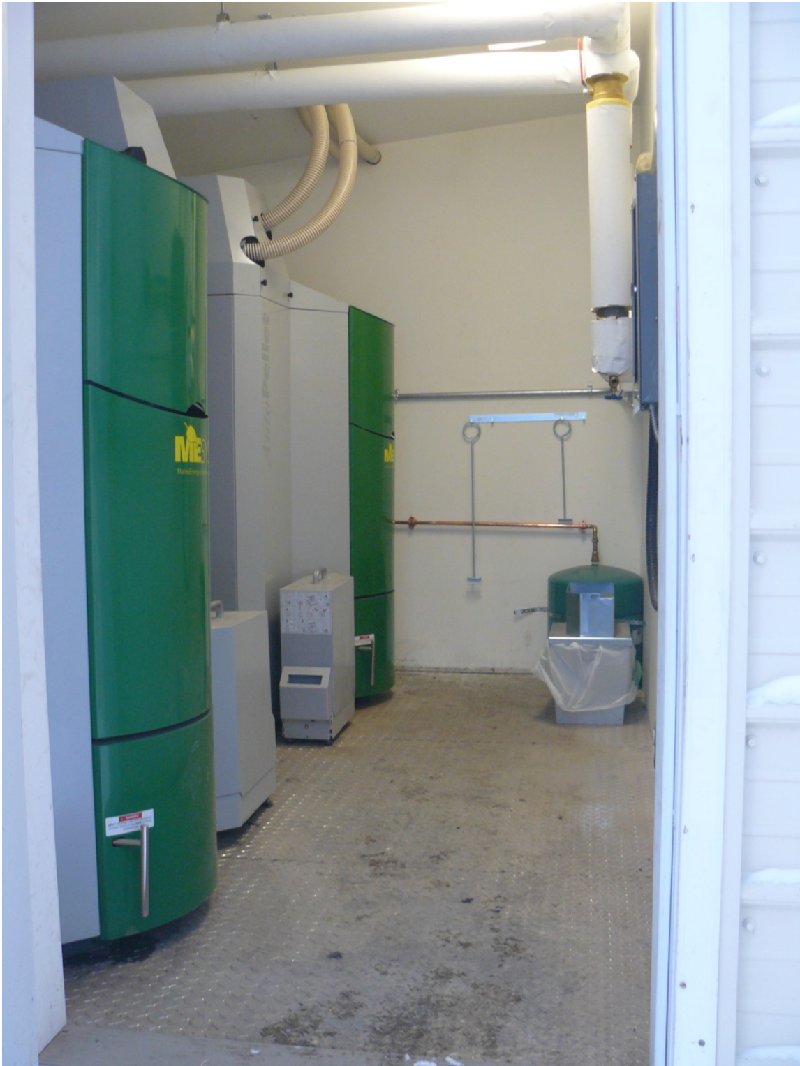
18 Figure 6: 2 56kW boilers in a cascade
