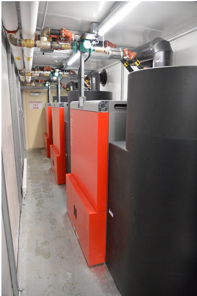
Figure 12: Staged Fröling biomass boilers
