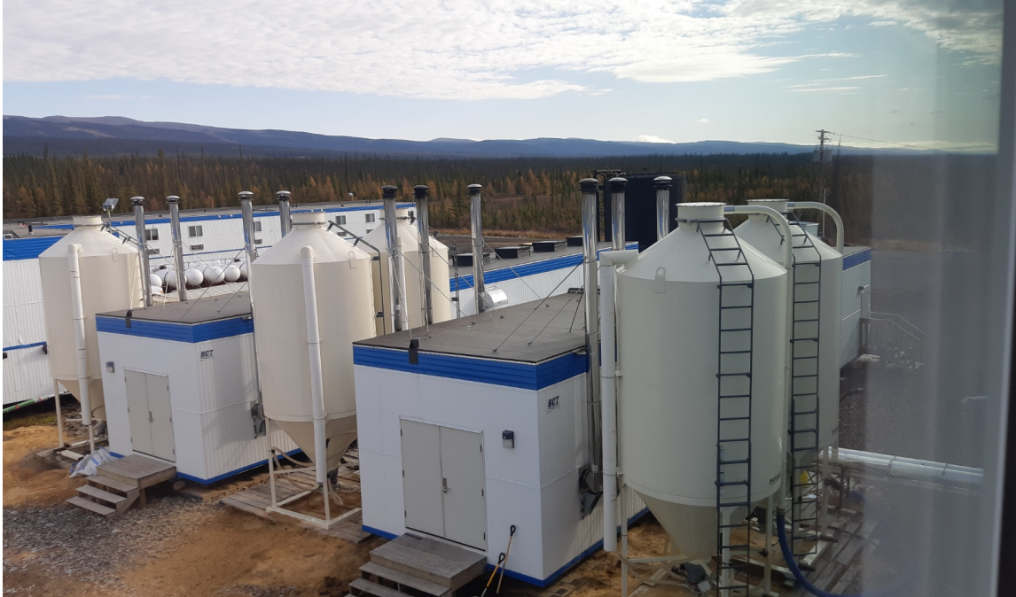
Figure 8: Boiler buildings housing pellet boiler cascades to heat a 93-bed dormitory for oil field workers in Norman Wells, NWT
