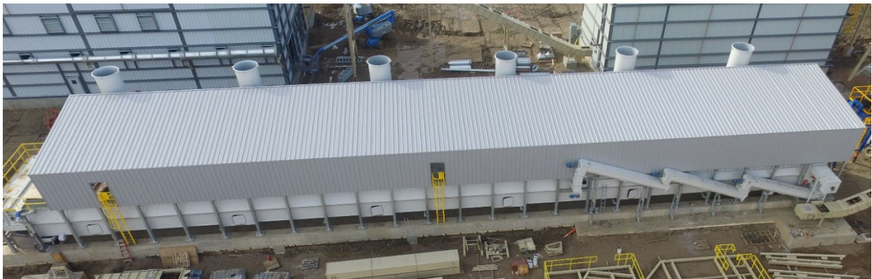
Figure D. 4. Prodesa Indirect-heated Belt Dryer
