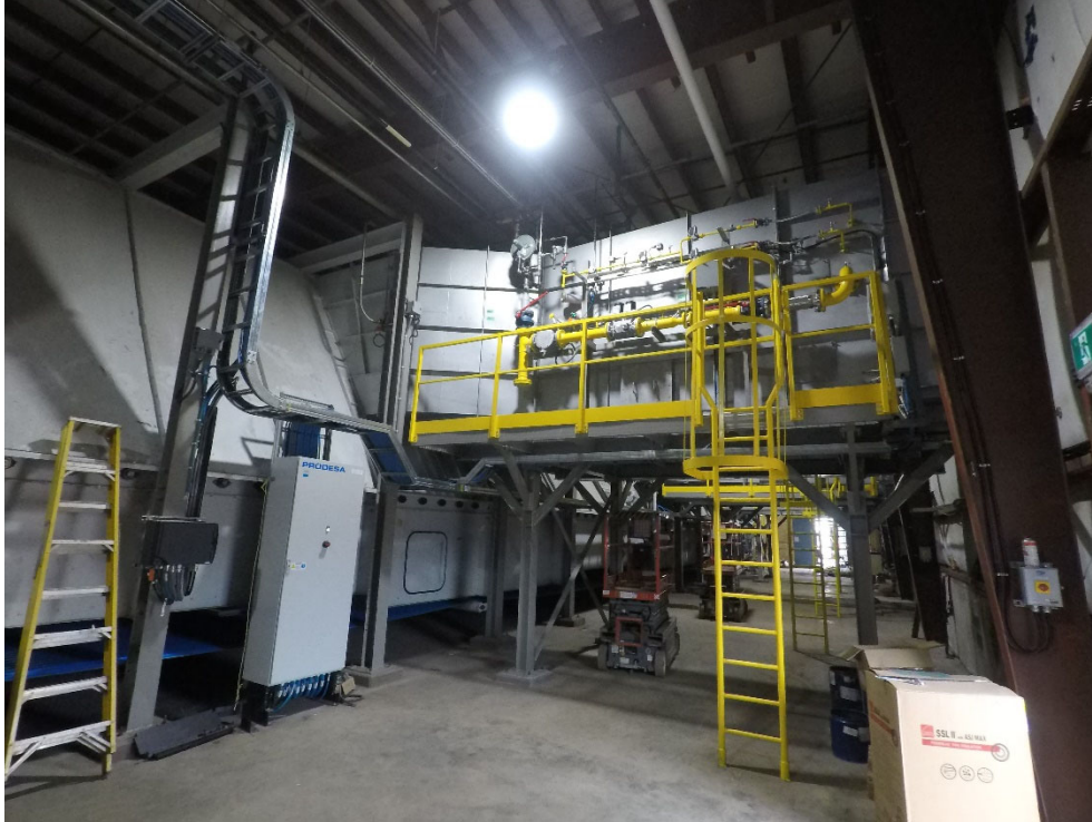
Figure D. 3. Prodesa's Direct- heated Belt Dryer (Skeena Bioenergy). View of the burner channel
