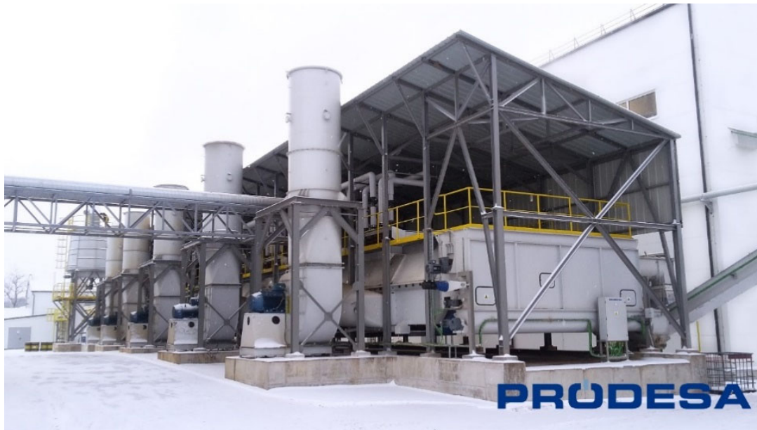
Figure D. 5. Prodesa Indirect- heated Belt Dryer
