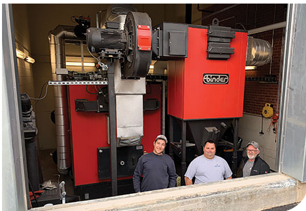
Serge Mallet (middle) responsible for mechanical/electrical systems and buildings maintenance at the CCNB-UDM Shippagan Campus seen here with colleagues Sebastien Chiasson (left) HVC Mechanical and janitor Maurice Gagnon (right).
