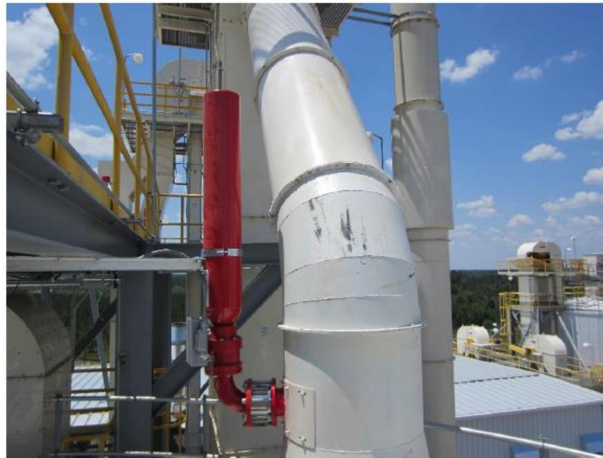
Example 1: Wood Pellet Bucket Elevator discharge chute isolated with chemical isolation
