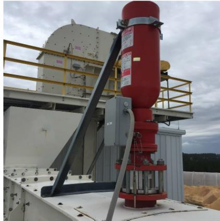
Example 2: Wood Pellet Bucket Elevator discharge conveyor isolated with chemical isolation
