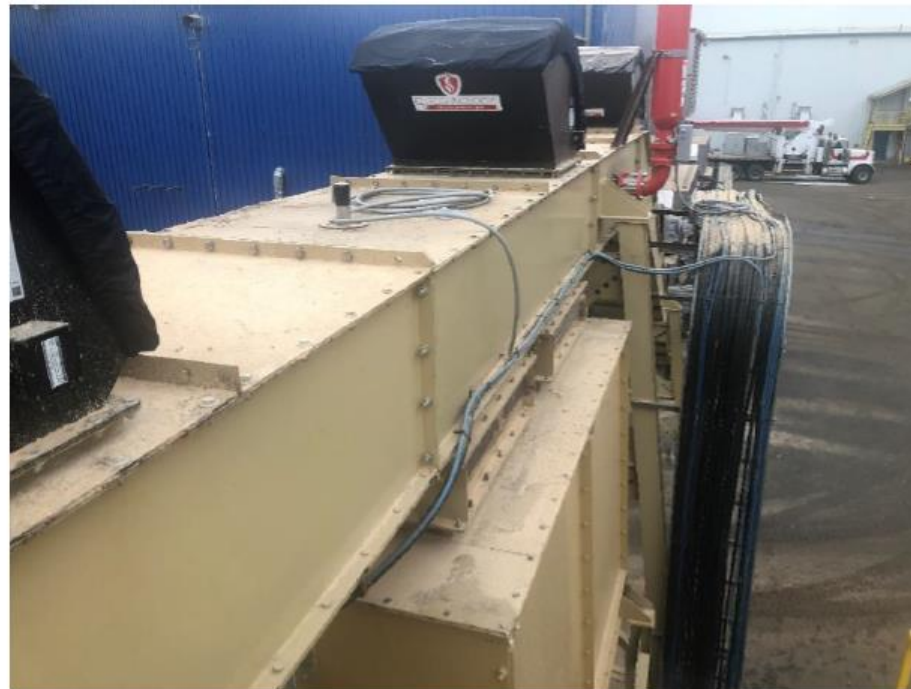
Example 1: Drag Chain Conveyor protected with flameless vents coupled with chemical isolation on the discharge chute connecting it to another conveyor
