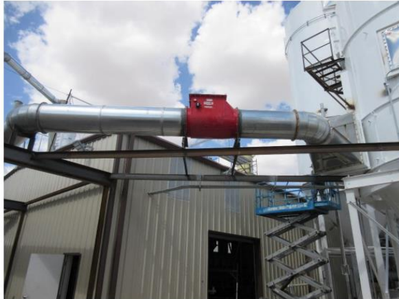
Example 2: Mechanical Isolation on the inlet line to a wood dust collector
