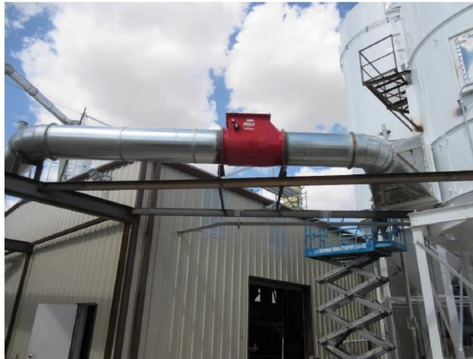
Example 2: Mechanical Isolation on the inlet line to a wood dust collector
